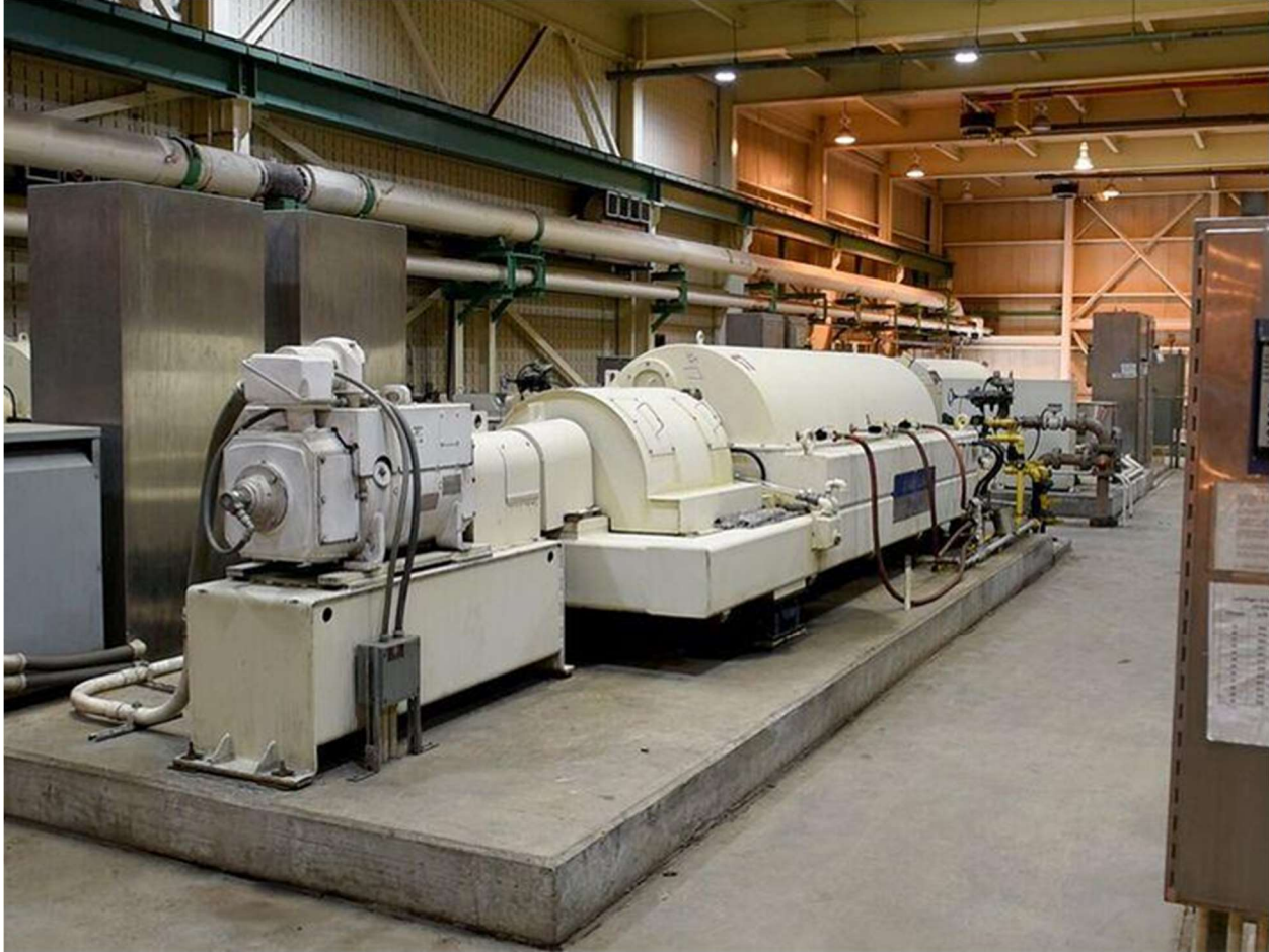
Exhibit 2. Centrifuge for dewatering sludge at the Stickney plant. Centrate is piped to another facility for processing while the cake drops to a conveyor on the lower level. Photograph courtesy of the MWRD.
